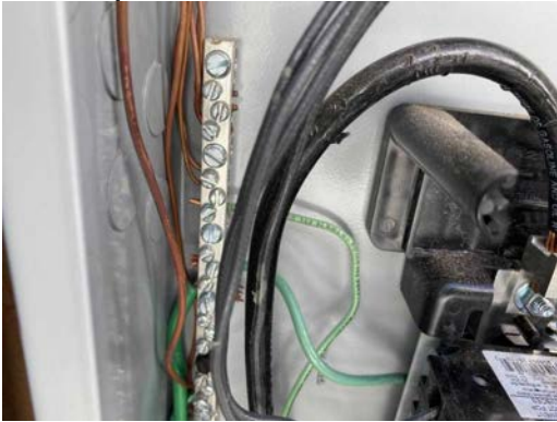
# 2 , Unit 2 Electric Panel
